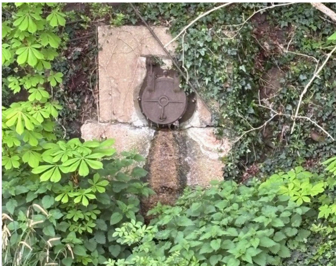
Raw sewage flowing into the brook
